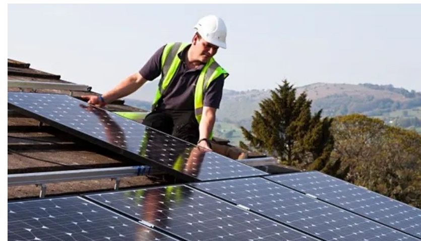
Example of PV panels installed on an existing roof. (Source: Alamy Stock Photo)
