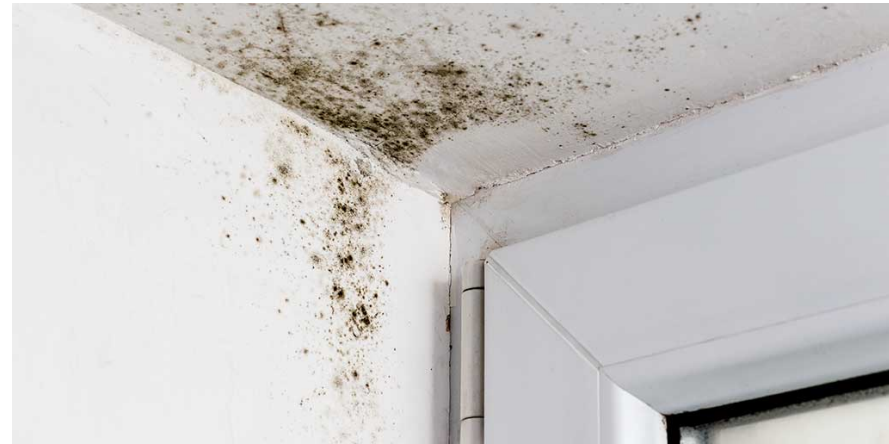
Example of mould growth in apartment ceiling due to moisture build-up and poor ventilation strategy
